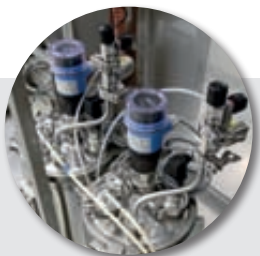
Chemical dosing system
