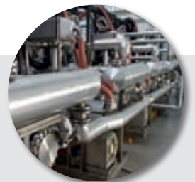
Water treatment supply
